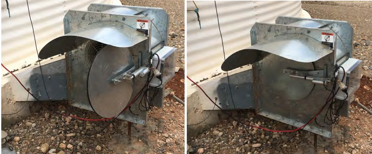
Figure 19. Electric actuated door to seal the fan inlet during periods of higher temperature. Door open (left) and door closed (right)
